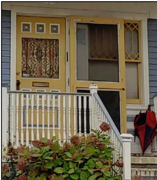
Appropriate wood door and screen door.
