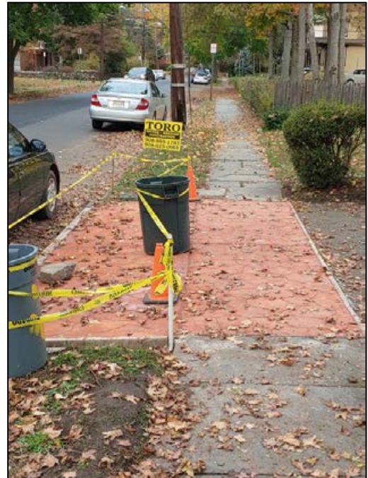
Inappropriate material change.
