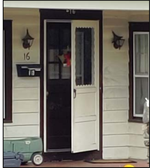
Inappropriate screen door.
