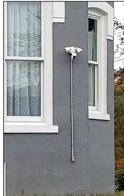
Inappropriate lighting fixture (LED floodlights).
