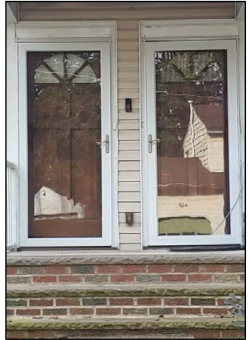
Inappropriate storm door.
