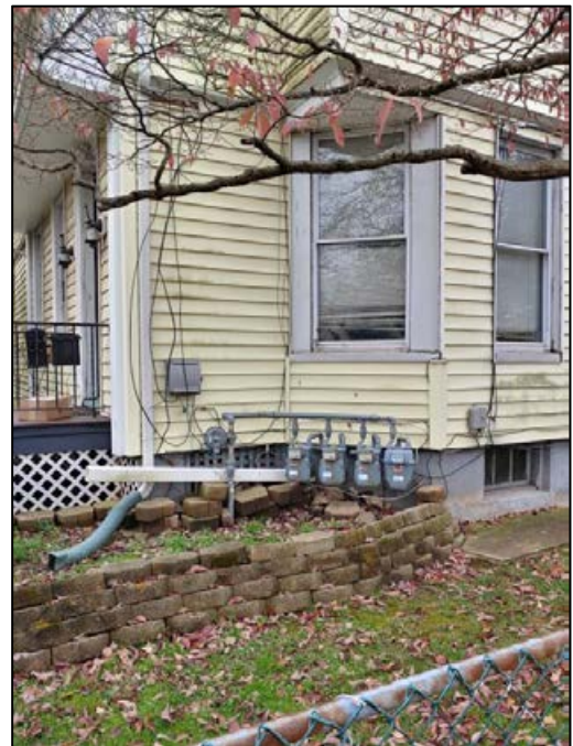
Inappropriate stone block wall in front yard.
