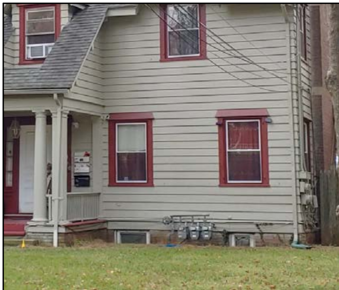
Concealed gas and electric utilities.
