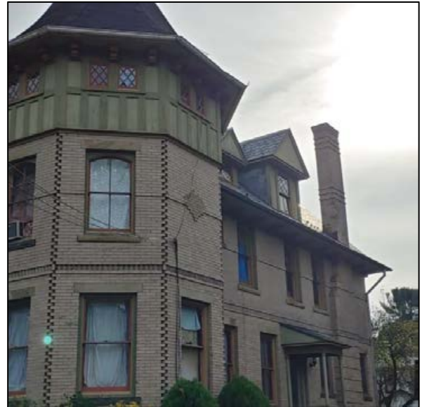
Wires attached to front elevation brickwork.
