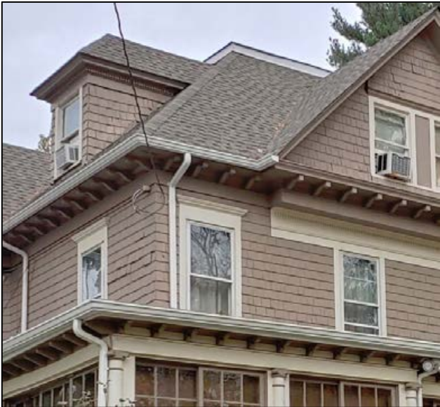
Wires attached under eaves and concealed.
