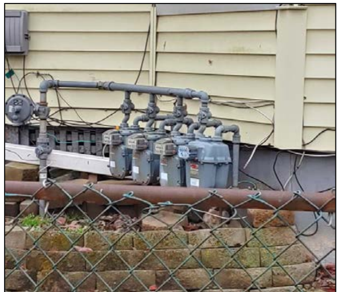
Exposed gas utility with no attempt at concealment.
