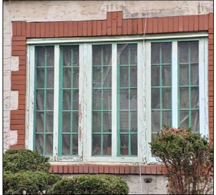
Poorly maintained wood casement windows.
