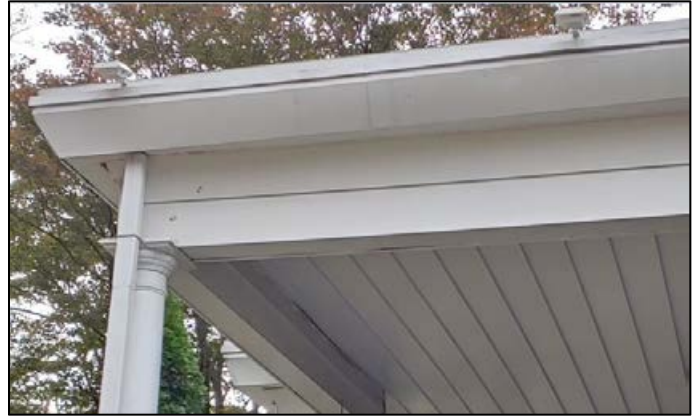
Inappropriate porch ceiling and floodlights.
