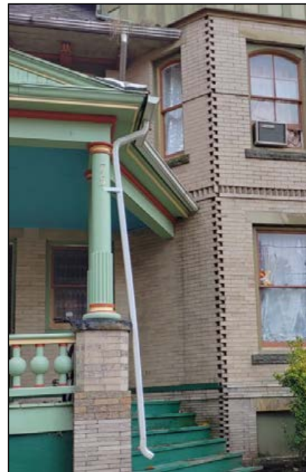
Inappropriate downspout placement.
