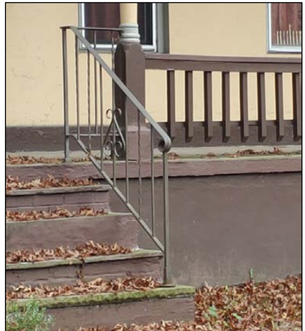
Inappropriate wrought iron railing
