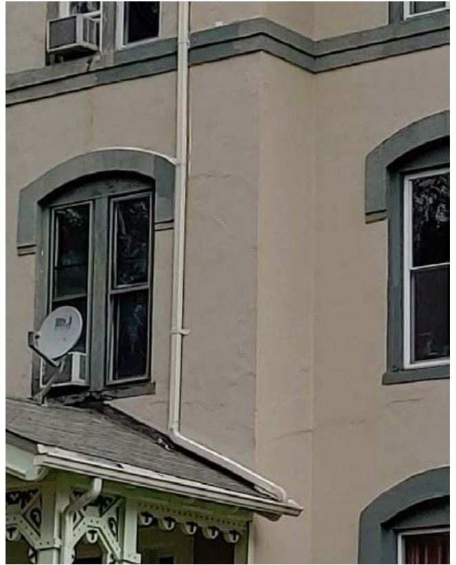
Inappropriate downspout treatment.
