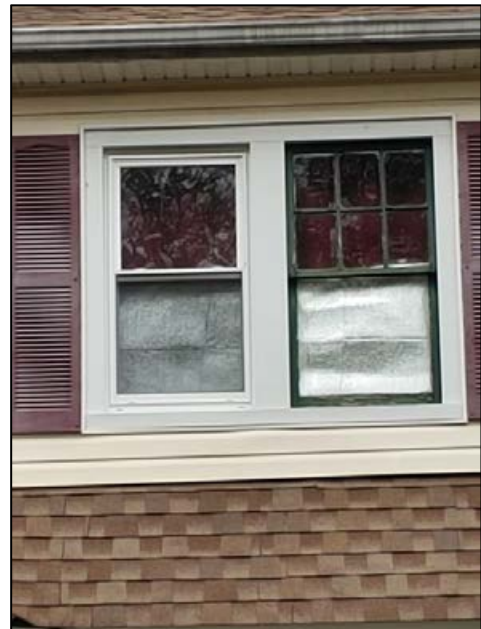
Replacement window (left) and original wood window(right).
