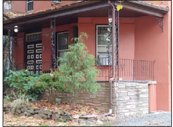
Inappropriate wrought iron railing and columns and brick veneer under porch.
