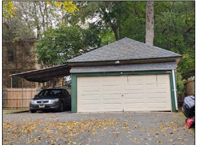
Inappropriate double-wide garage door.
