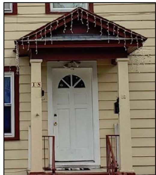
Inappropriate modern door with fanlight.
